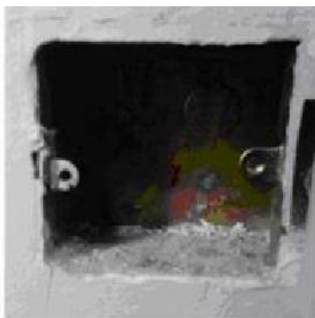
1. 86 Socket on the wall
