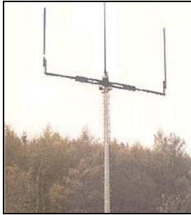
Omnidirectional base station with a single cell
